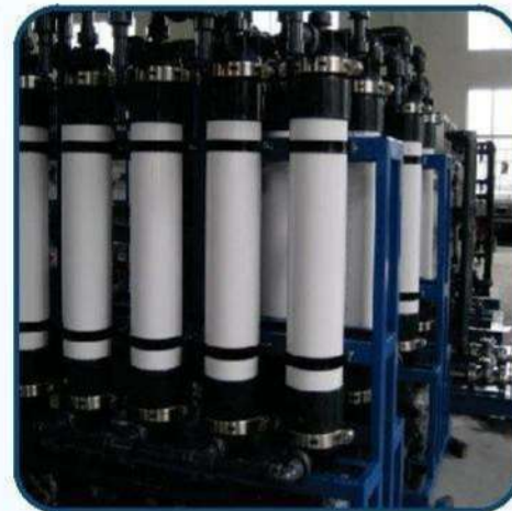
Ultra Filtration System
